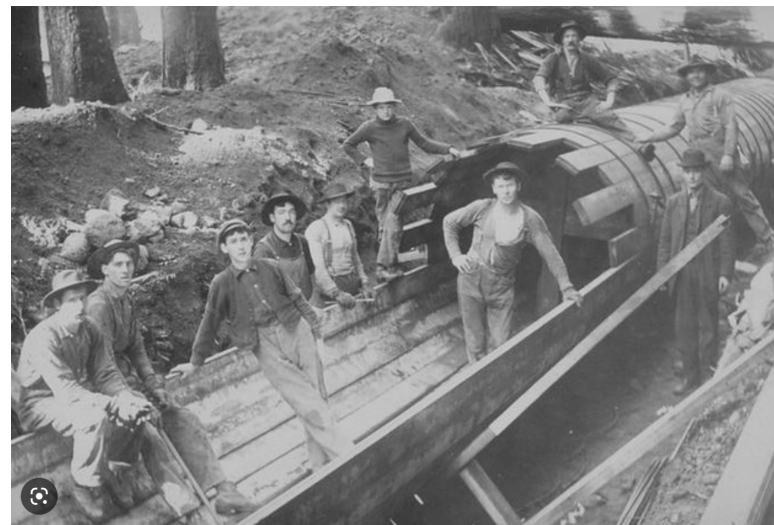
Workers constructing wood stave pipeline similar to those whose remains we see at Salisbury Mills, circa 1890, source: Flickr.
